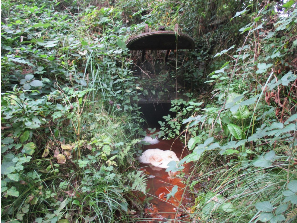
The mystery outfall pipe. Note flap that is always up, the foam and reddish liquid emerging.
