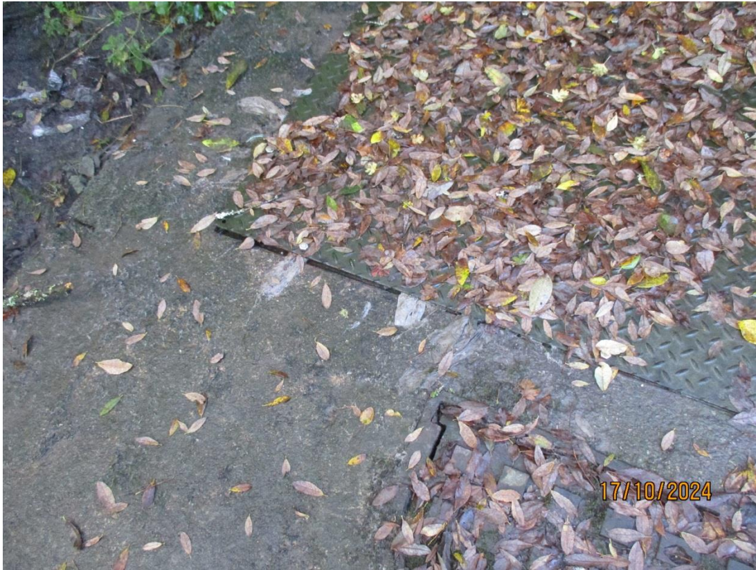
Metal plate presumed to be part of a CSO tank near the Molinnis Stream.
